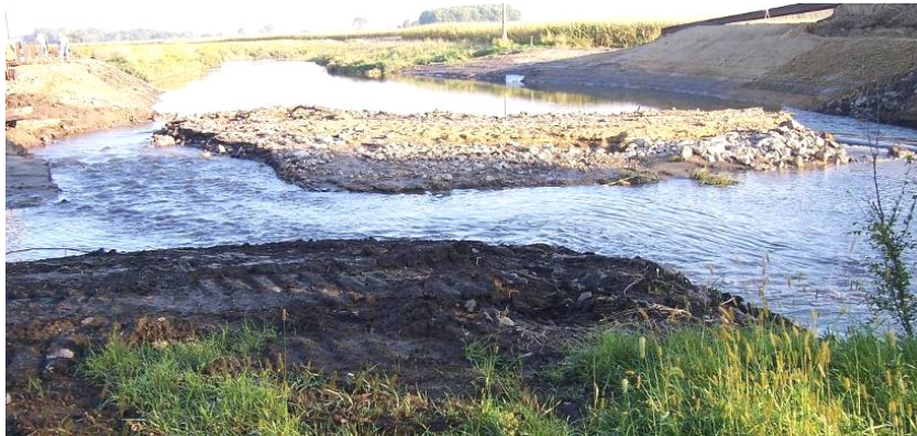
Figure 108. Washed out access road, September 15.
