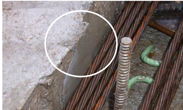
Figure 86. Concrete obstruction in Channel 1.
