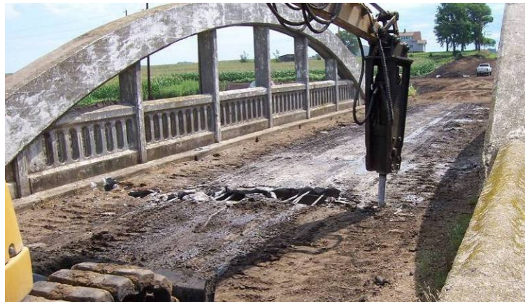
Figure 104. Breaking apart the Marsh Arch bridge deck with a back hoe, July 24.
