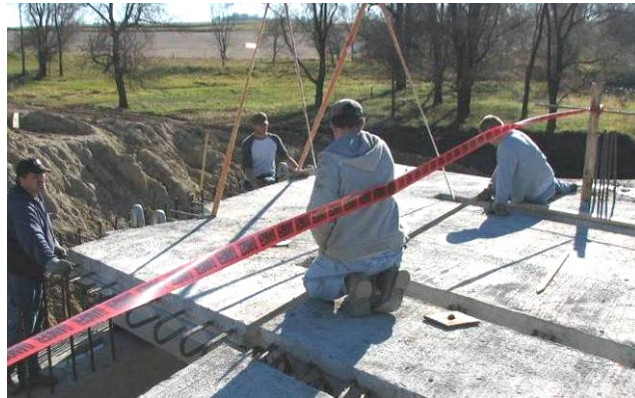
Figure 134. End panel being placed at the east end of the bridge, November 8.
